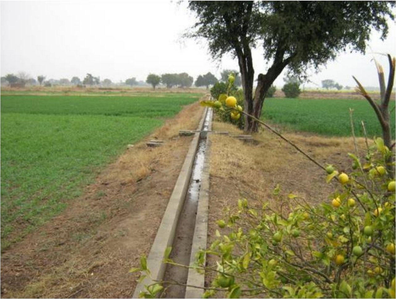
picture: irrigation drain
